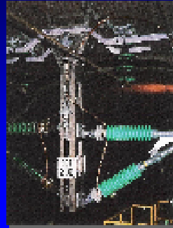
Shin-kanon Undersea Tunnel Trolley Wire Frame
