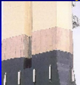
Sheathing for ice protection for Trans Tokyo Bridge is made of titanium bonded to steel
